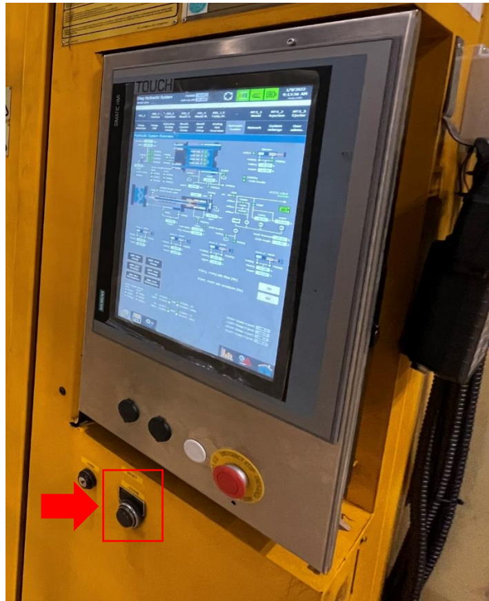
Figure 64: Front gate interlock push button location
